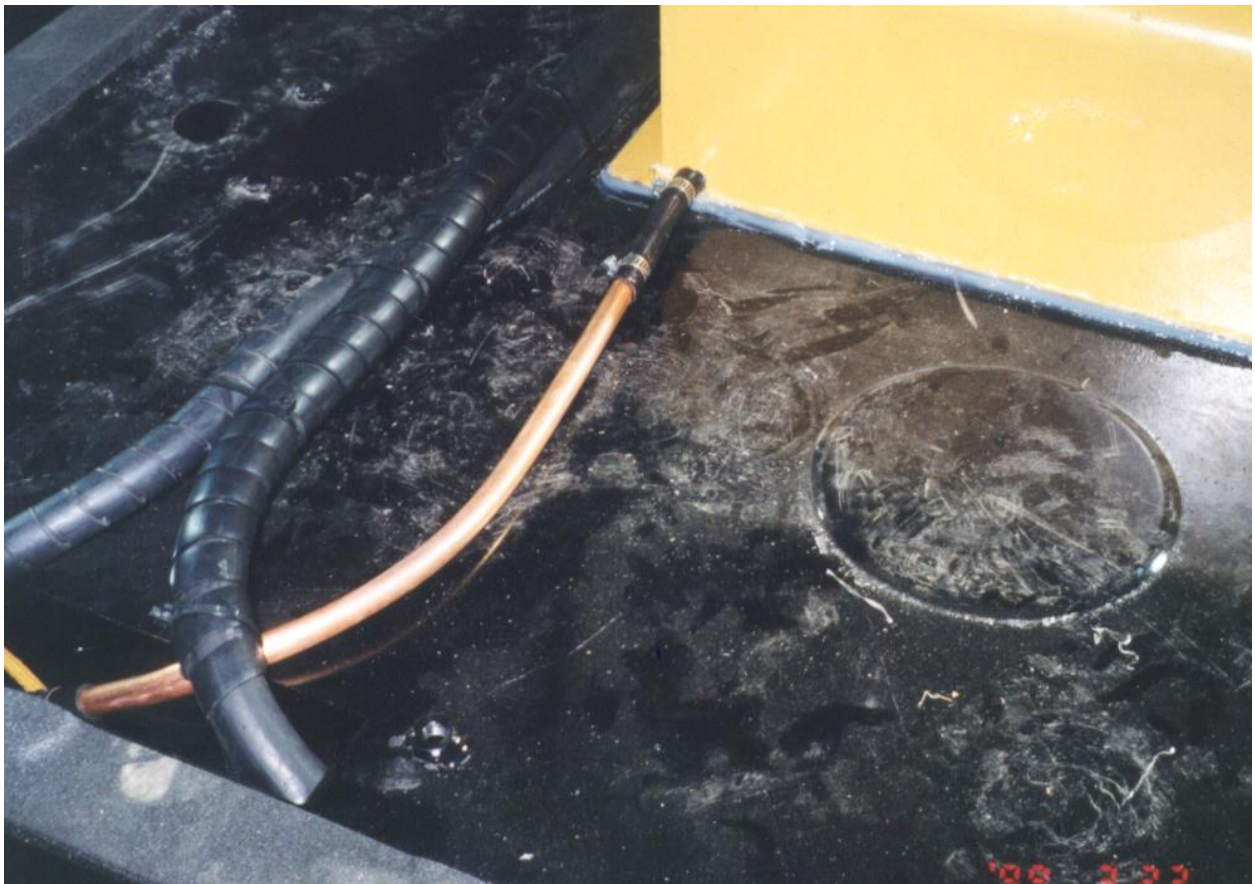
Drain tube and hoses running through front rectangular opening in roof.
