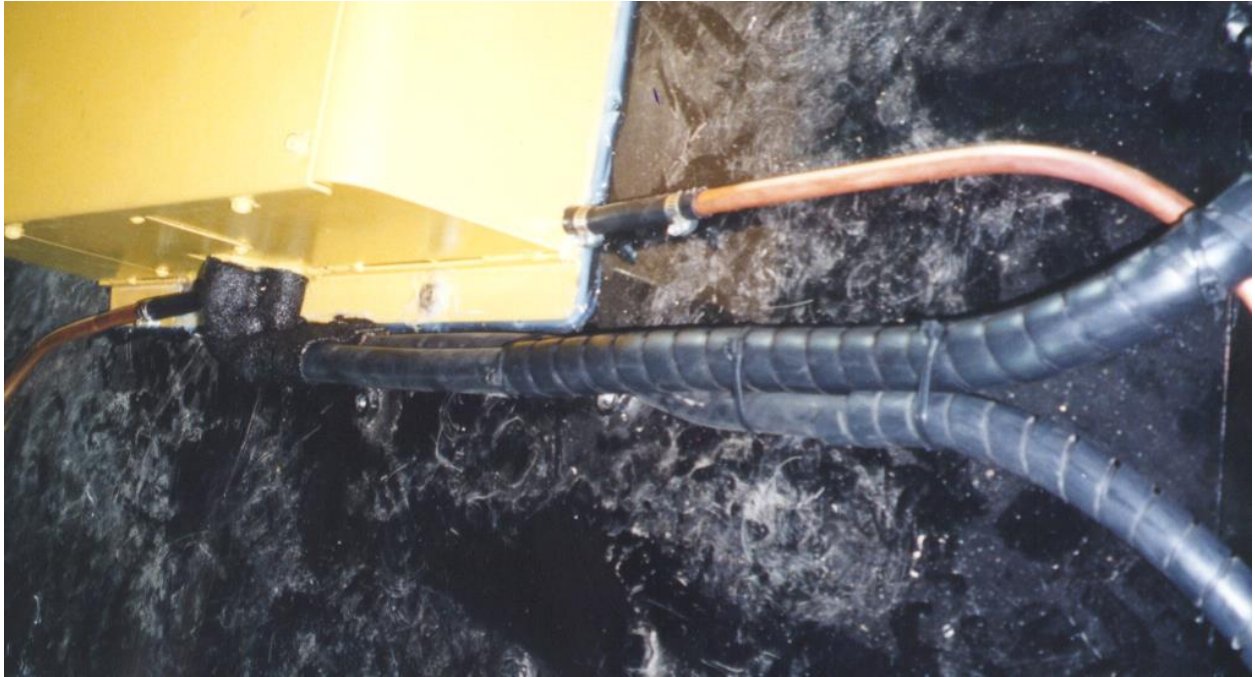
Hoses on roof to evaporator inlet and outlet fittings.
