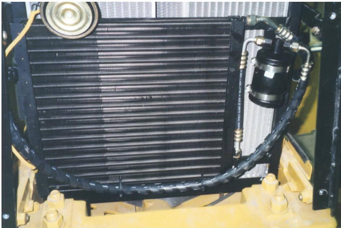
Hoses at condenser.
